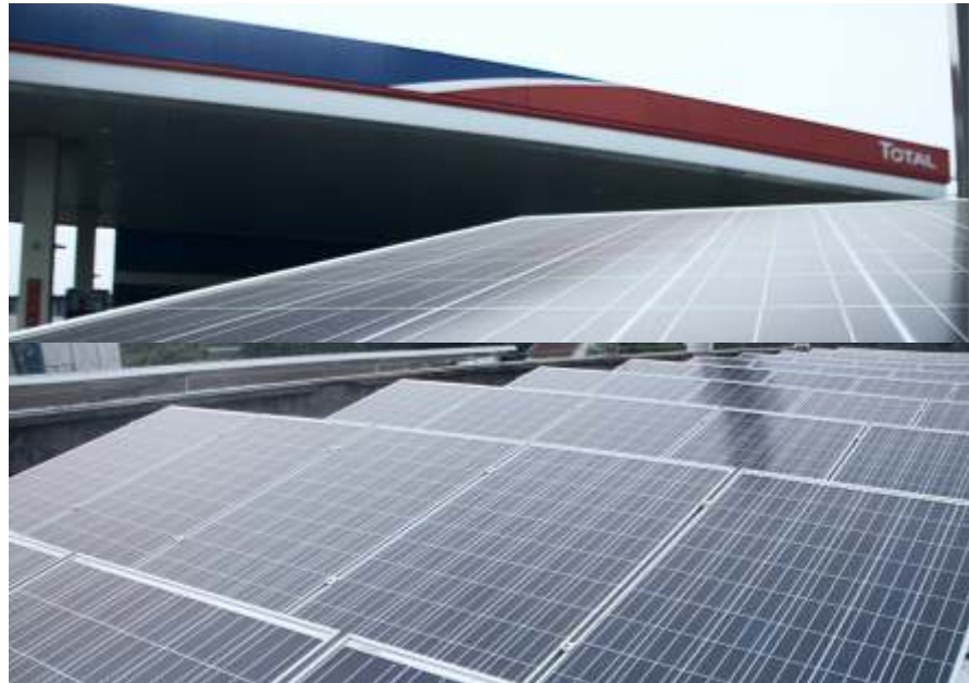
30kW, Petrol station
