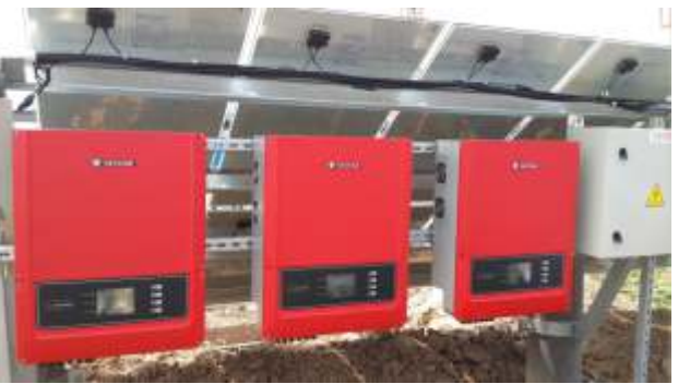
250kW, Shangdong, China
